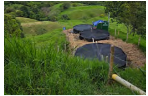
These tanks sit just outside of town and supply water for the company's projects. See that hill at the top right? Believe it or not, water is pumped UP that mountain—and then two more beyond it!—to reach the furthest of the projects. It takes three pumps total, with eight people watching the system 24/7.
