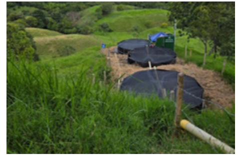
These tanks sit just outside of town and supply water for the company's projects. See that hill at the top right? Believe it or not, water is pumped UP that mountain—and then two more beyond it!—to reach the furthest of the projects. It takes three pumps total, with eight people watching the system 24/7.
