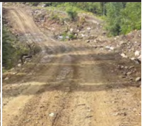
Upgrade of all-season access road for its flagship Kenbridge Nickel project in Ontario.
